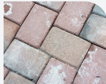
Efflorescence paving Block
