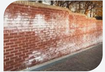
Efflorescence brick wall
